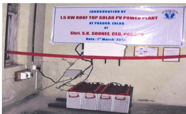
Solar PV Power Plant
